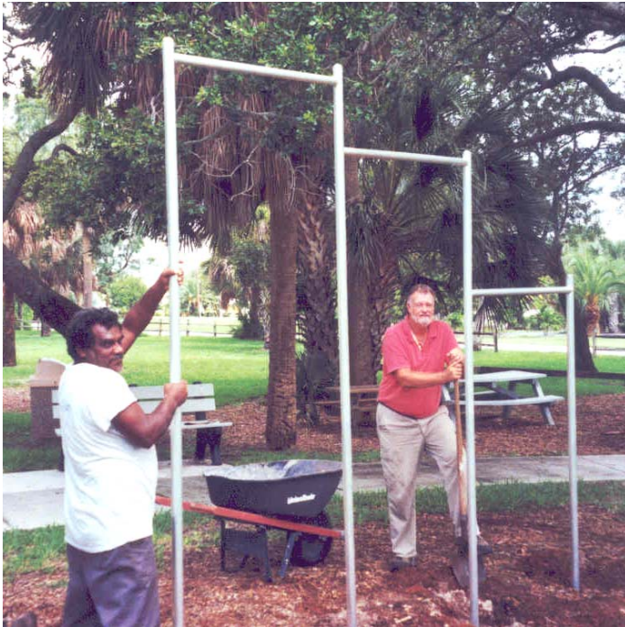
Public Works personnel Isaiah Cepeda and Ron Cassidy install new chin-up bars in Orlando Park. The previous set of chin-up bars deteriorated and was removed last December.
