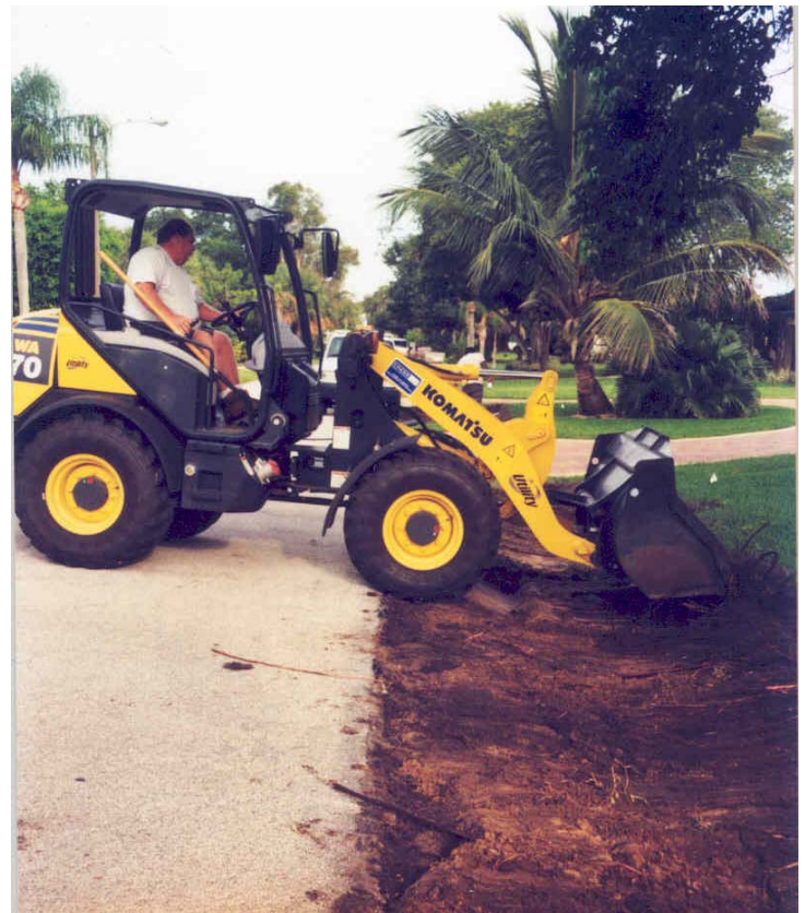
John Howard, with the Public Works Department, constructs a swale at 310 Miami Avenue. Swales are a commonly used stormwater practice recommended to treat runoff to reduce pollution. Property owners desiring to have a swale installed in the street right-of-way in front of their property should contact Public Works Director Ron Cassedy at 984-5224.
