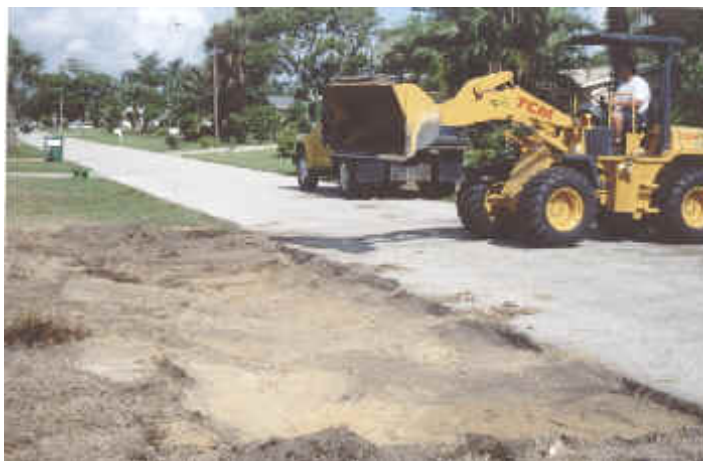
Town Public Works personnel continue efforts to capture water run-off in street side swales. This swale was installed recently on Eighth Avenue
