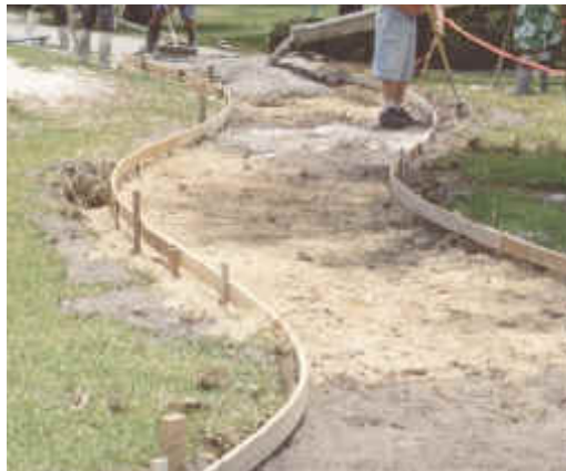
Don Bo, Inc. installs a sidewalk around the play area in Orlando Park
