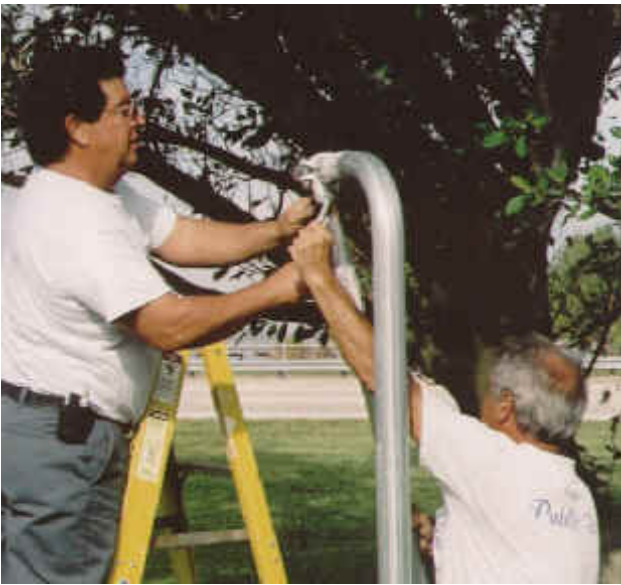
Public Works employees Tony Yacovino and Tony Breglio install an adult swing in Douglas Park. The Parks, Recreation and Beautification Committee recommended the purchase of two swings with a second one to be installed in Orlando Park
